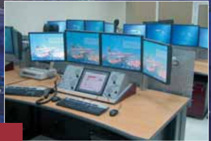
QATAR Qatar Airways, OCC, Doha
